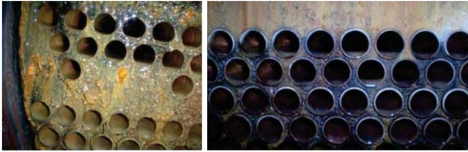
Figure 7.1: A tube-in-shell heat exchanger shown before the application of Hydropath (left), and after (right) where not only has the limescale been removed but magnetite has begun to form as a hard black deposit.
